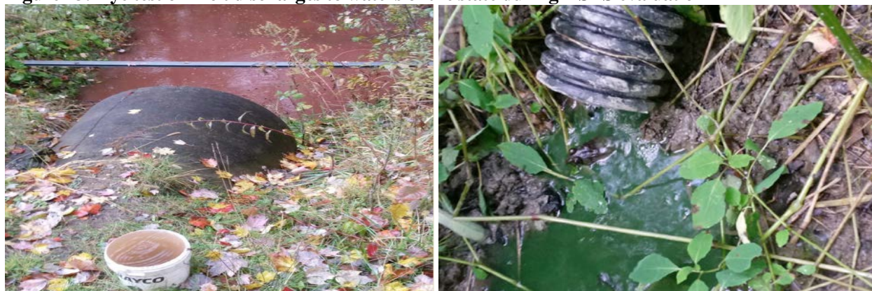
Figure 13: Dye test of illicit discharges to waters of the state during HSTS evaluation
